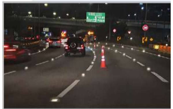
9. Installation in Gangbyeonbuk-ro by Seoul Metropolitan Facilities Management Corporation
